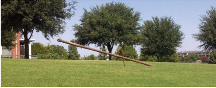
A drill stem surfaces near the Baylor Law School after boring under the Brazos River. The drilling will provide a path for installation of optical fiber connectivity between the main Baylor campus and the BRIC.
